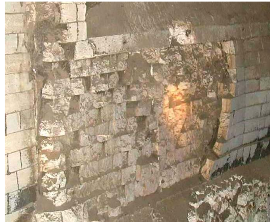
“alkalibursting” on the wall of a cement cooler; big areas fall off due to irreversible expansion
